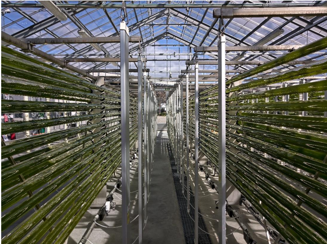
Figure 20. 750L tubular photobioreactors at the algae pilot in Mongstad during production of Microchloropsis gaditana .
